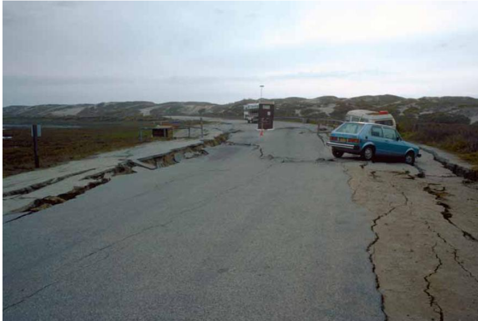
Fig 1.5: Ground failure due to liquefaction, Loma Prieta earthquake
