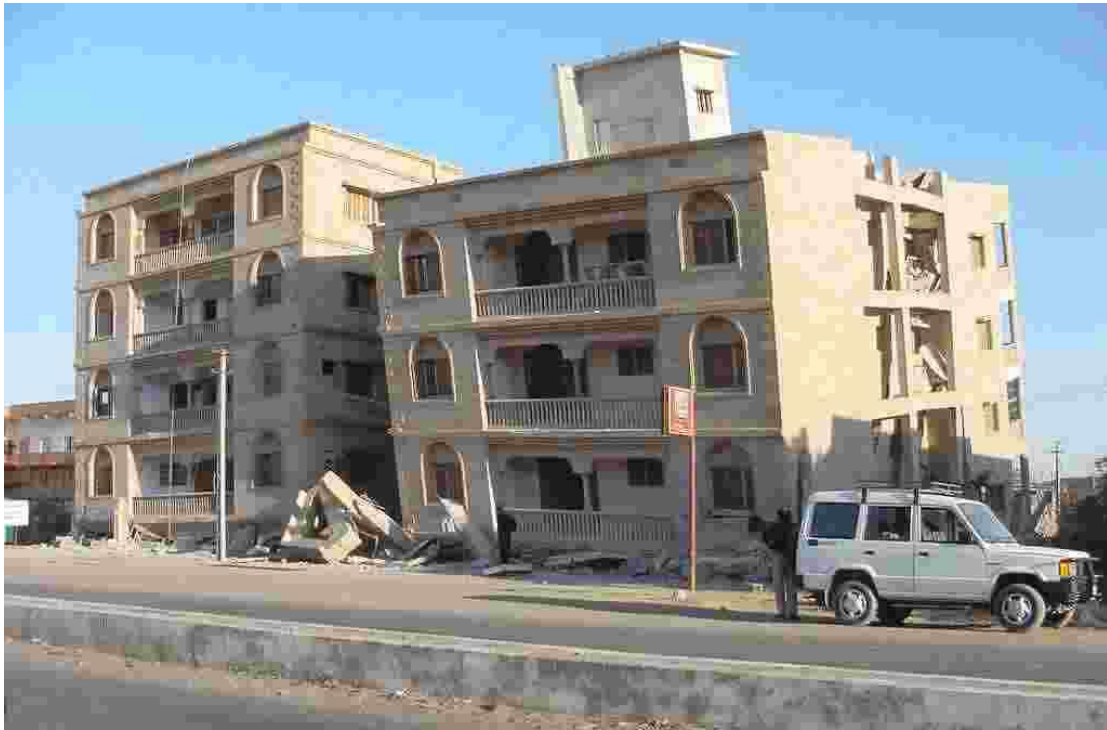
Fig 1.1: Ground storey collapse of a 4-storey building at Bhuj in Gujarat, India.
