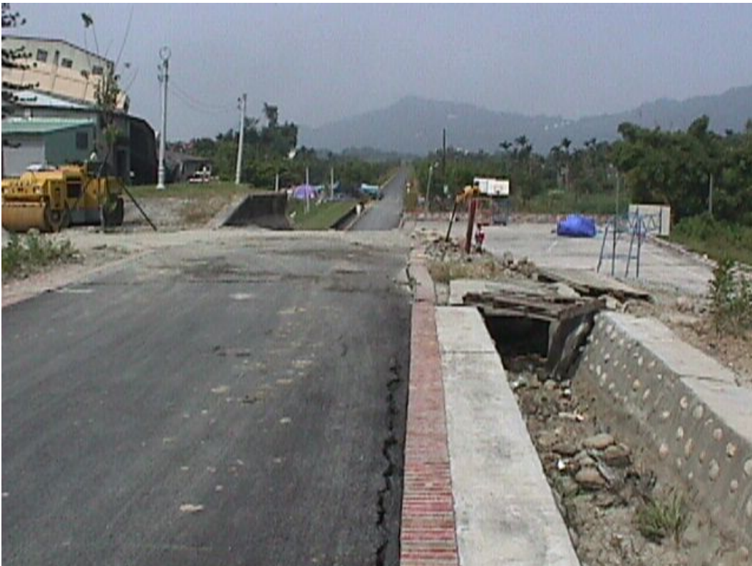
Fig. 1.82 - Chichi (Taiwan) earthquake of 1999. The fault cuts diagonally across the picture. Almost all movement was thrust, with less than 1 m left lateral slip.
