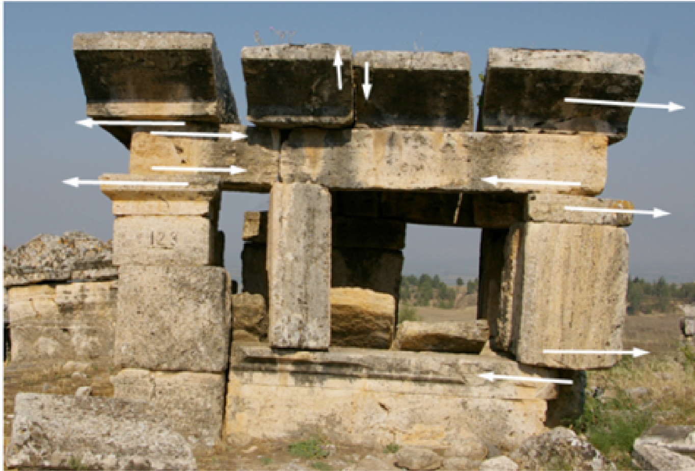
Fig. 2.12 - Ruins of a tomb in Hierapolis, an ancient city in Turkey founded around 200 B.C. and abandoned after an earthquake in 1534. Many offsets can be observed between the different blocks: although gravity may be a primary driver of this tomb deformation, perhaps occasional seismic shakings contributed (taken from Callan Bentley in AGU Blogoshere).
